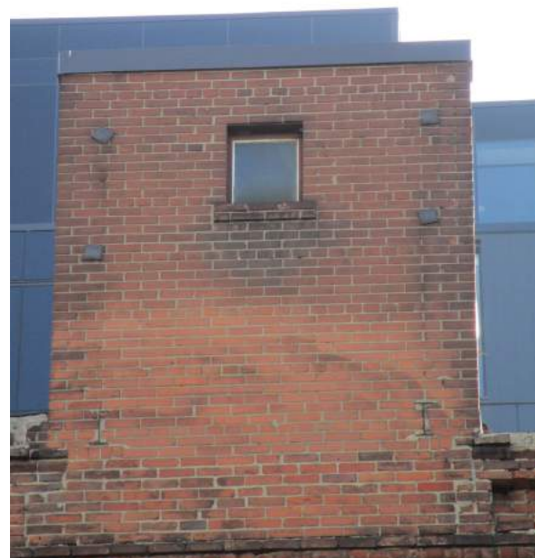
Clockwise from top left: removed entryway and modified door; windows, masonry sills and brick detailing (typical; southern bays); roof access/penthouse addition; parapet (typical).
