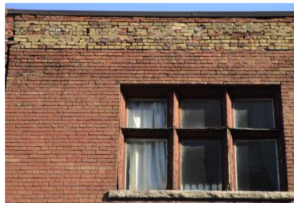
Top to bottom: south elevation (general), south elevation masonry (typical); parapet and masonry sills).
